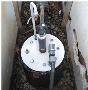
Cooper Well w/ New Head and Electrical Wiring
