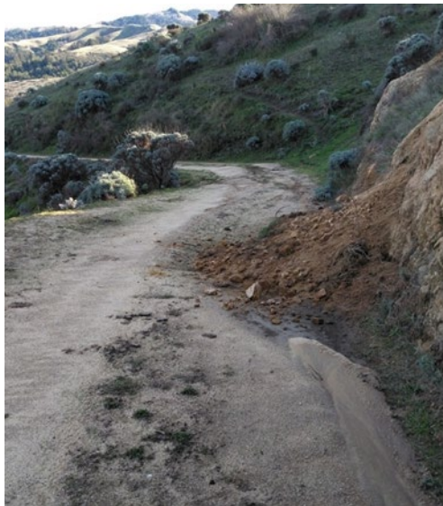
Minor landslide at Chamise Ridge
