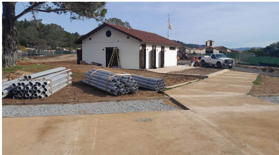
Restroom facility with Granitecrete permeable pathway (and Event Pad in foreground)
