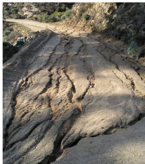
Soil erosion along PC Trail
