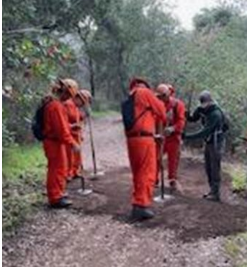
Garza Canyon Trail drain dips
